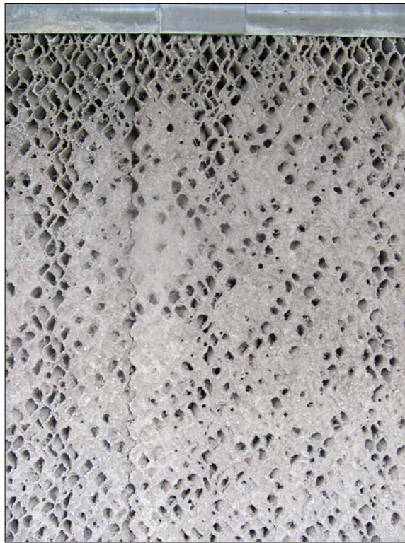
Figure 1. Cool cell pads clogged by mineral deposits.
