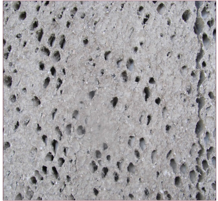
Figure 3. Mineral buildup clogs cool cell pads.
