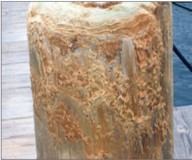
Figure 2. Salt killed piers, pilings, seawalls, and other marine structures are common.
