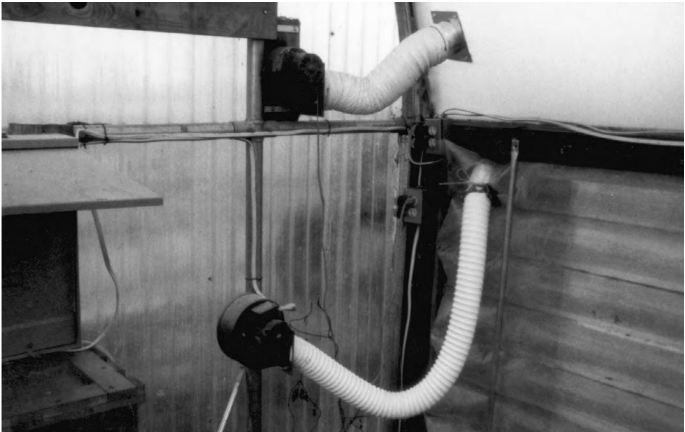
Small squirrel-cage blowers (1/4 or 1/2 HP) can be used to inflate between the two layers of plastic covering the greenhouse. It is important to use outside air for this purpose so that condensation does not collect between the layers.
