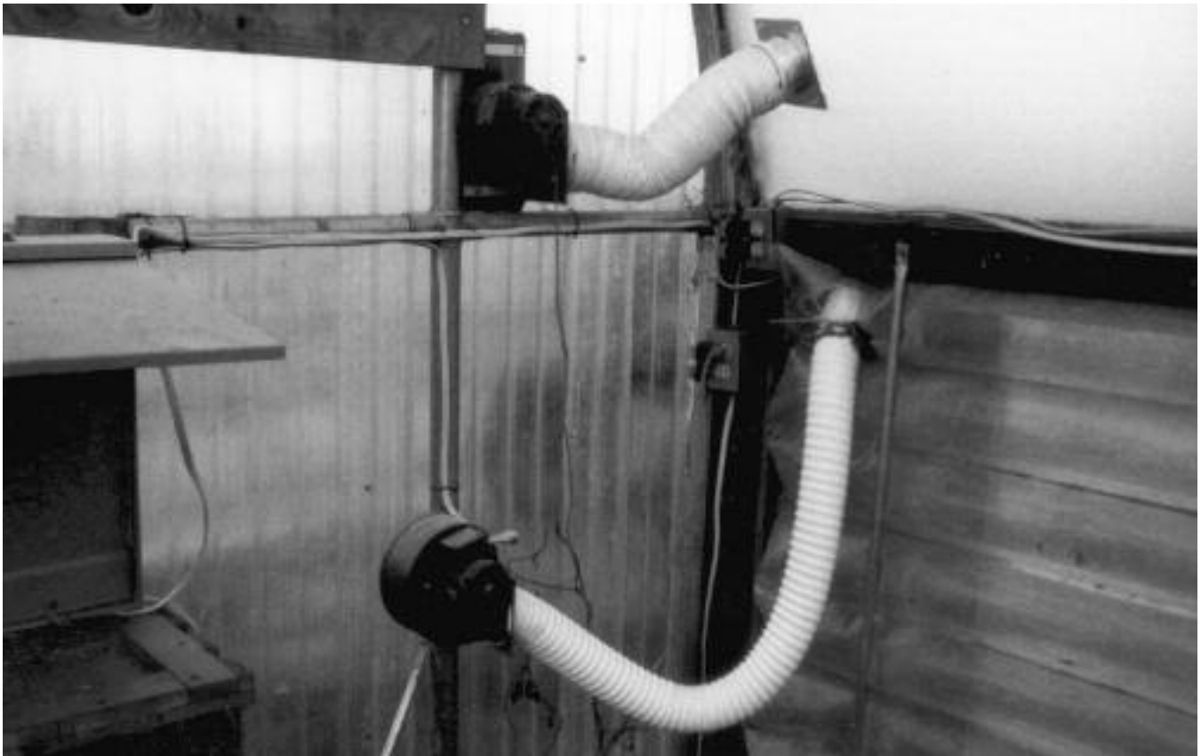
Small squirrel-cage blowers (1/4 or 1/2 HP) can be used to inflate between the two layers of plastic covering the greenhouse. It is important to use outside air for this purpose so that condensation does not collect between the layers.
