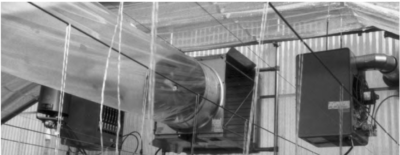
Traditional fan jet systems are commonly used to distribute heat produced by heaters and to recirculate inside air when the heating system is not in use.
