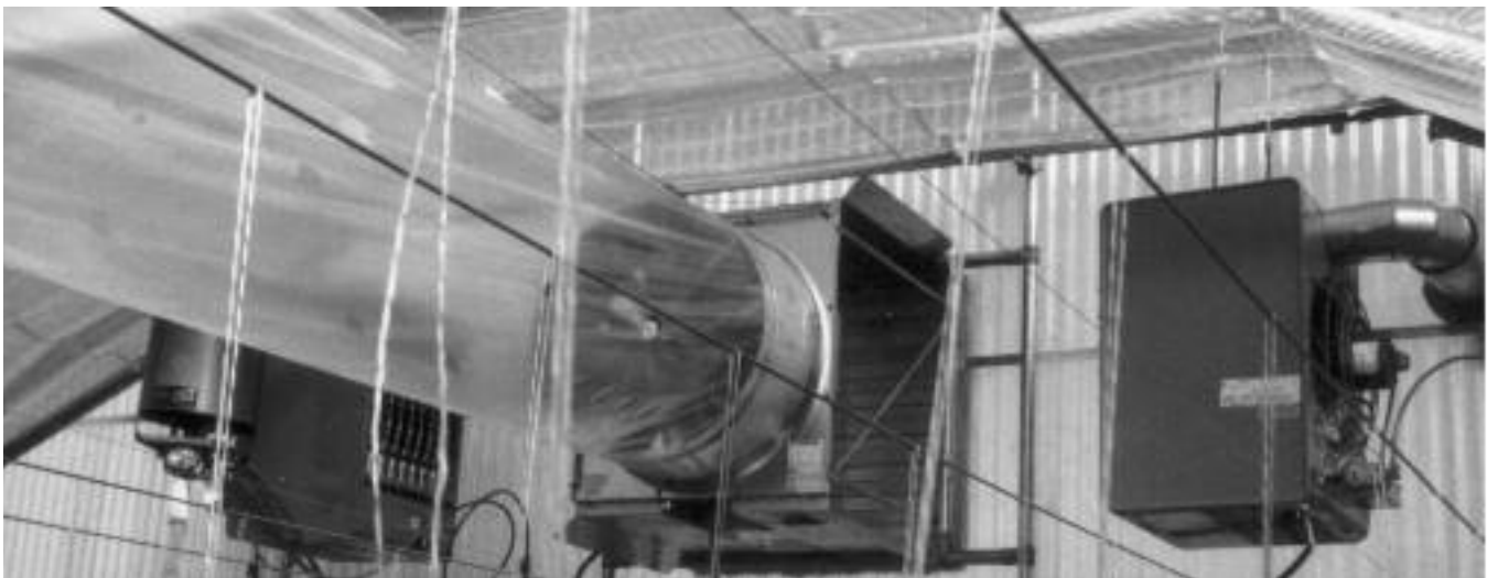
Traditional fan jet systems are commonly used to distribute heat produced by heaters and to recirculate inside air when the heating system is not in use.
